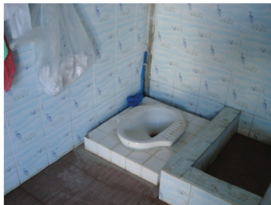
Toilet had lock inside
